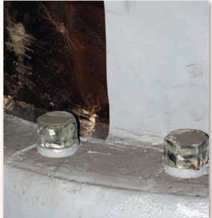
An additional layer of EPDM rubber was applied to protect the insulation where the pneumatic gun was used.
