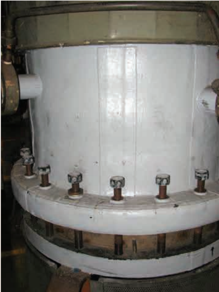
The 2 mm insulation thickness was the maximum that could be used given the space required to screw the bolts using a pneumatic gun.
