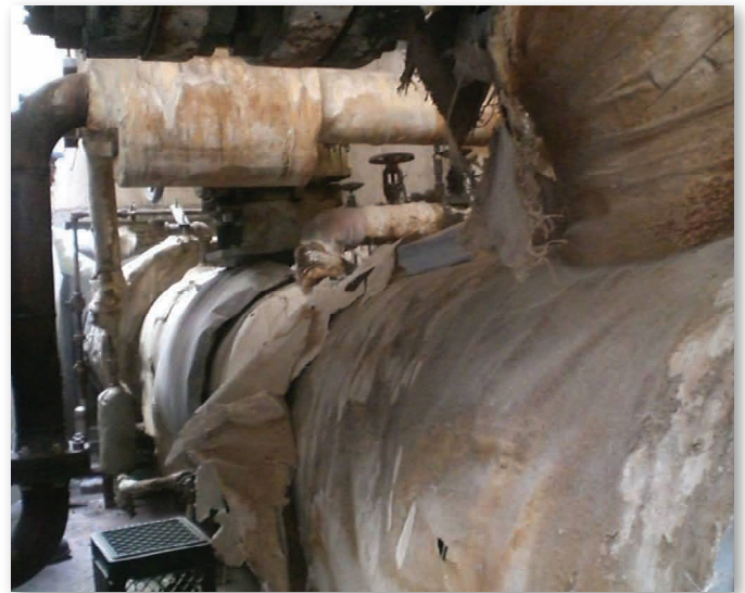
Old insulation in vault
