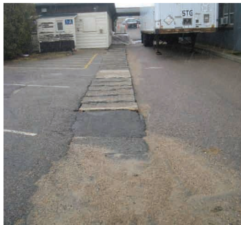
Heat from steam line warms trench covers to 64°F; ambient temperature 34°F
