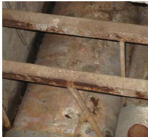
Insulation under cladding severely degraded over time; degradation exacerbated by trench flooding events
